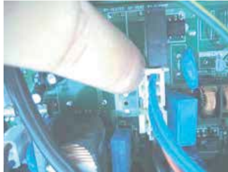
** Indoor PCB Drain Pump Connector (Check Electrical Input; Marked as CN-DPUMP)
